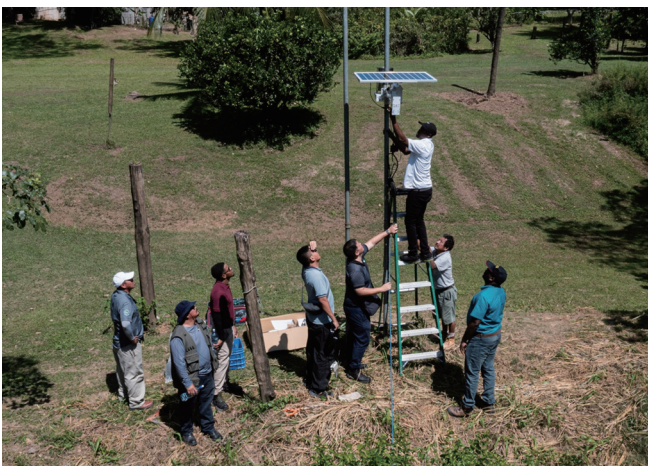
▲ Figure 2-37 With the Project for Flood Warning Capacity Improvement for the Belize River Basin, TaiwanICDF dispatched experts to guide local technicians in repairing hydrological monitoring station equipment
